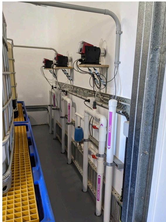
Figure A.5.2 Chemical dosing pipework (for example) is well labelled.
