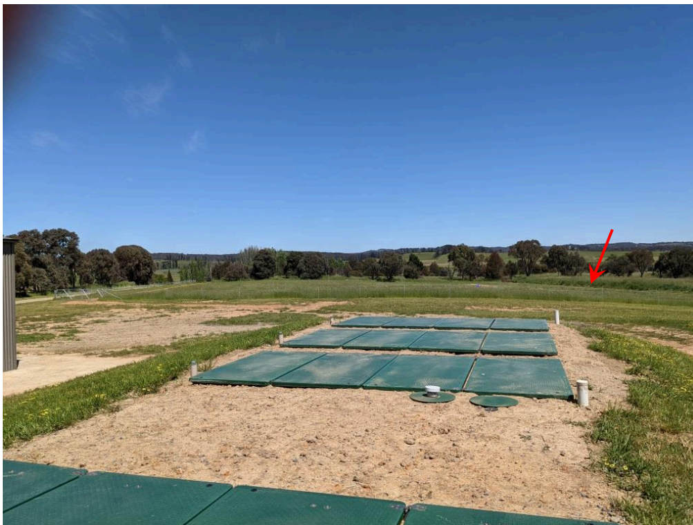
Figure A.9.2 Treatment plant construction area showing line of one of the diversion drains (arrowed) in background.
