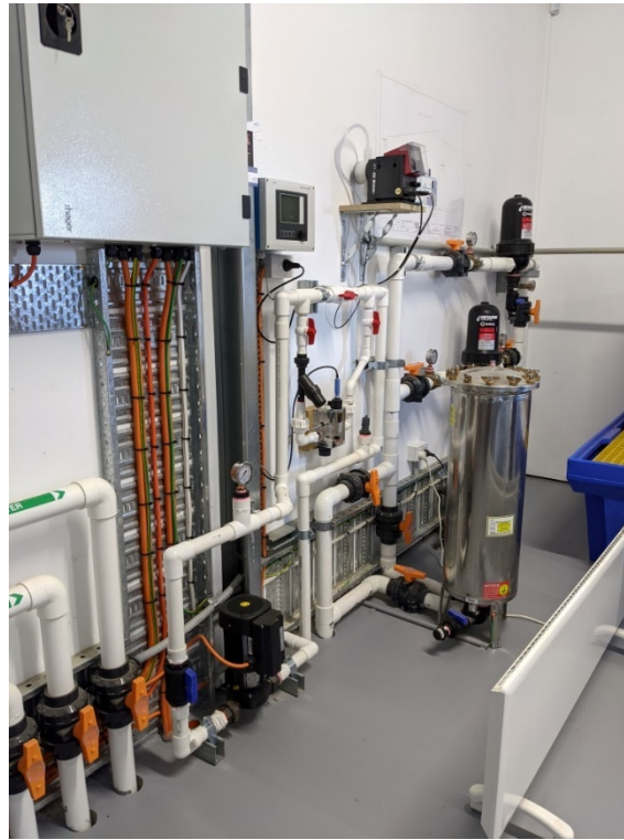
Figure A.3.3 Chlorine dosing pipework and equipment, and Helminth filter.
