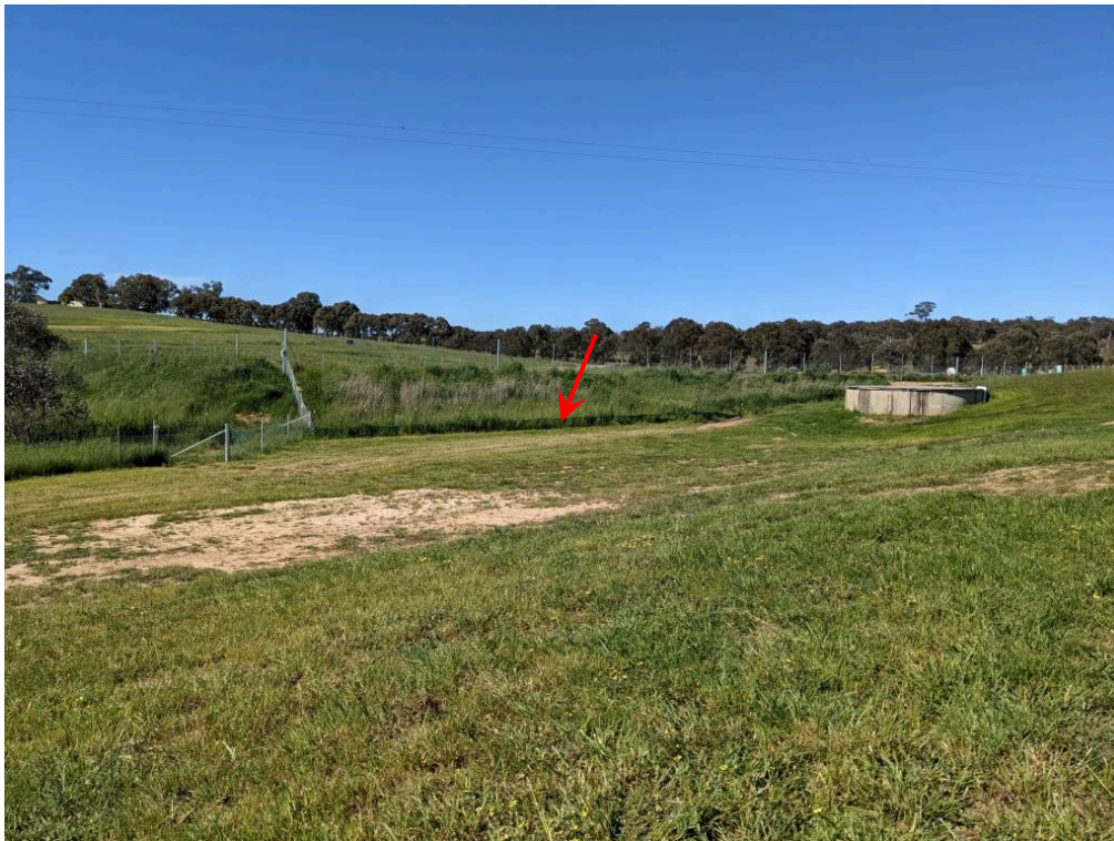
Figure A.9.5 Construction area adjacent to treatment plant looking towards wet weather storage dam. Silt fencing (arrowed) in background; re-established grassing in foreground.
