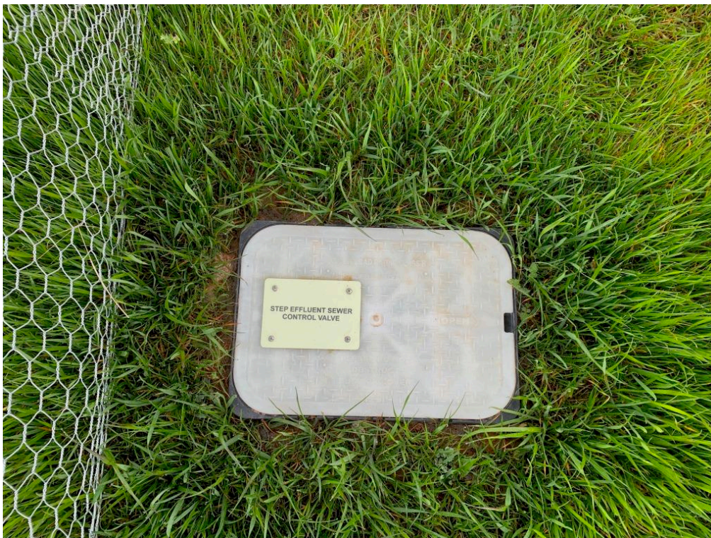
Figure A.3.2 Property connection point and isolation valve covers are clearly labelled.
