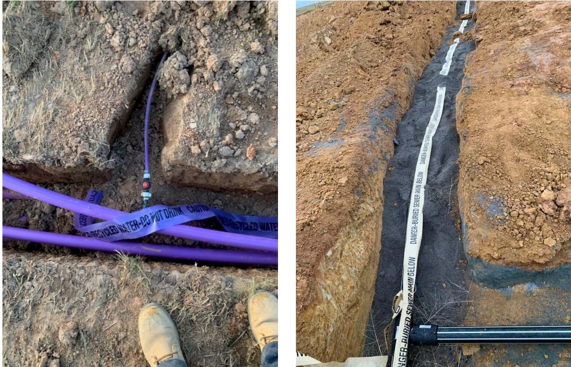
Figure A.5.1 Recycled water pipework in the irrigation field is coloured lilac; pressure sewers are cream striped and installed under maker tape with tracer wire.
