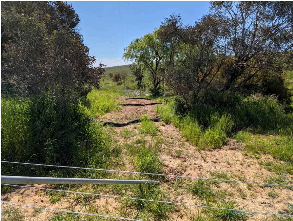
Figure A.9.3 Waterway downstream of wet weather storage dam (located to the right). Shows silt socks along flow path and stone silt trap in background
