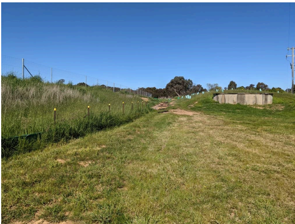
Figure A.9.4 Construction area adjacent to wet weather storage dam (embankment at left) showing silt fencing to the left and silt socks in background.
